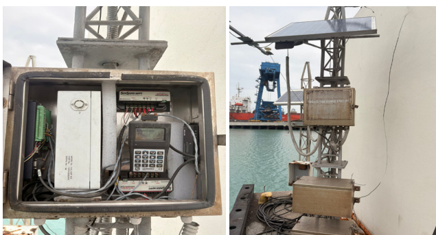
Automatic Tide Gauge Monitoring System
